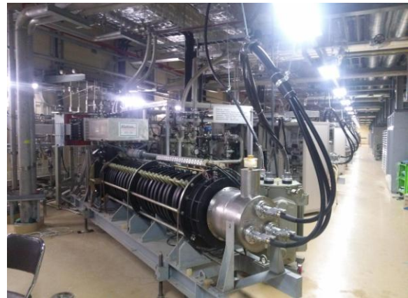
Figure 2: RF systems installed in the klystron gallery
