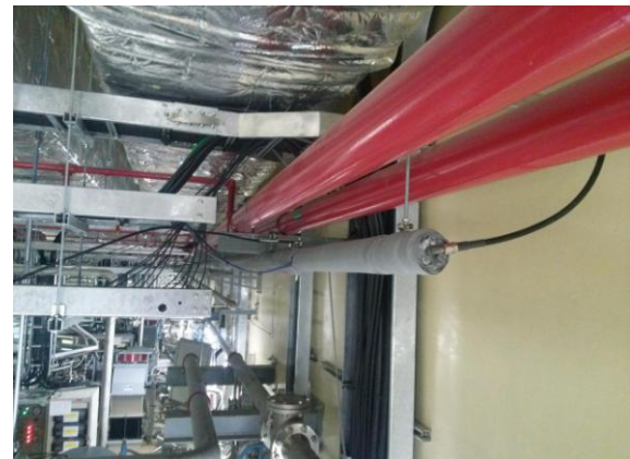
Figure 3: Temperature-controlled RF reference line
