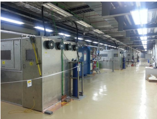
Fig. 1. Installed modulators in 3 rd floor of accelerator building
