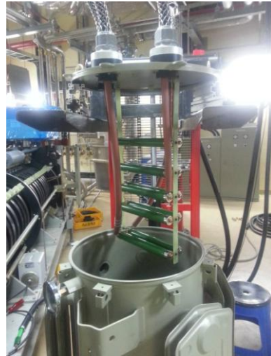
Fig. 2 Inside of diving resistor vessel for RFQ klystron
