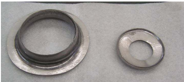
Figure 5. Broken part of beam-pipe transition.
