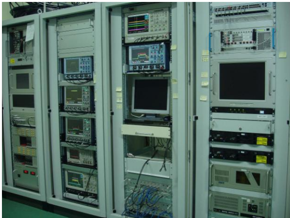
Figure 5. RF power distribution and measurement system
