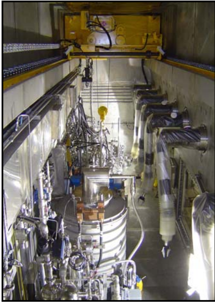
Fig. 2. Inside View of the ACPF Process Cell
