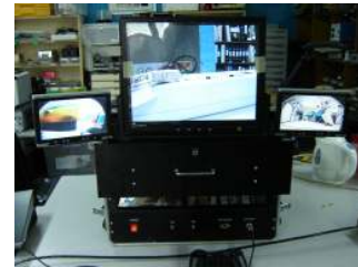
Figure 8. Monitoring and control console.
