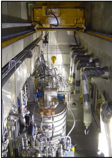
Fig. 2. Inside View of the ACPF Process Cell
