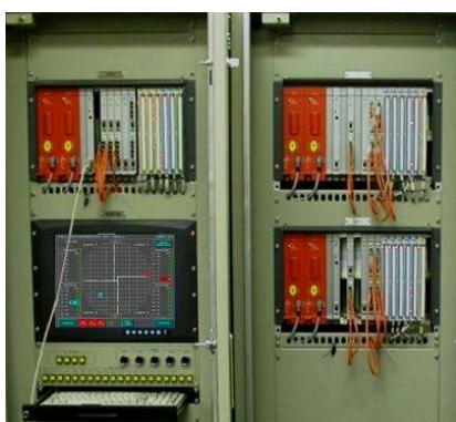
Figure 2. 1 Channel QIAS-P Cabinet
