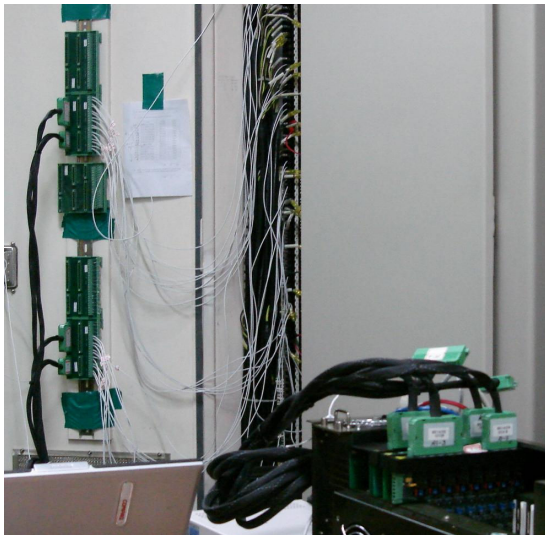
Figure 2. Connection between NSSS control system and performance verification tool using A/D converter
