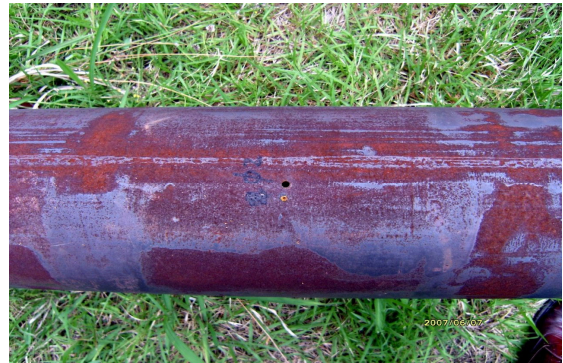
Figure 2. A Hole with a diameter of 5 mm fabricated in a mock-up pipe.
