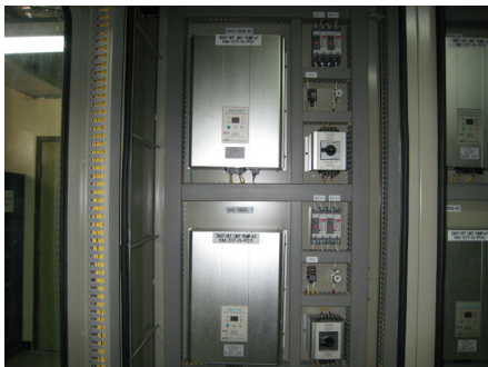
Figure 4. Installed sag compensator
