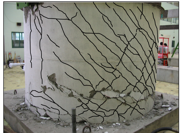
Figure 4. Failure view after SFMT of PCCV test model
