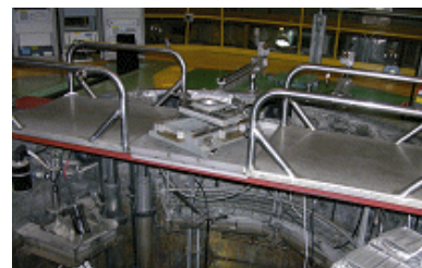
Figure 2 The measuring equipments installed on pool
