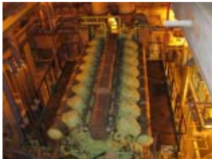
Fig. 1 Emergency Diesel Generator
