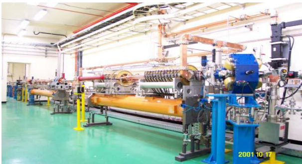
Figure.1: A photo of PLS-PNF electron Linac tunnel.
