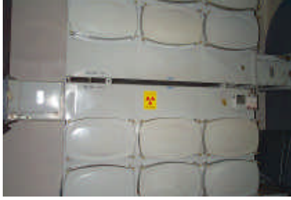
Fig. 2 HEPA filter casing.
