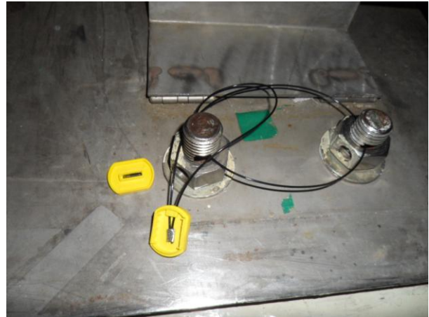
Figure 3. Seal at the Spent Fuel Transfer Canal Gate at LWR
