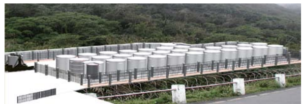
Fig. 1. Dry storage facility in Chinshan, Taiwan
