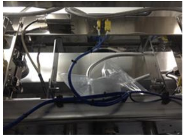
Fig.1. Salt transfer equipment heated by electrical control.
