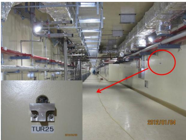
Fig. 1. An align network in the tunnel.
