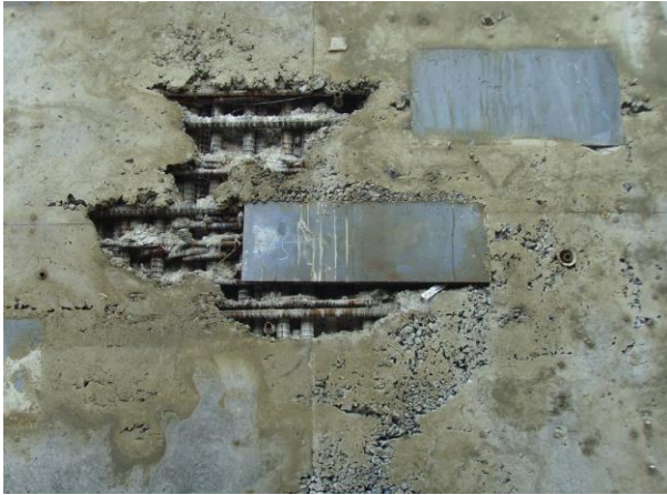
Fig. 2. Concrete honeycomb around embedded plate
