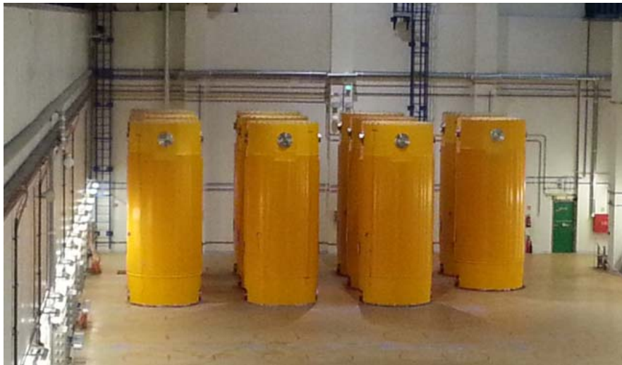
Fig. 7. CASTOR® 1000/19 in the interim storage facility at Temelin/Czech Republic
