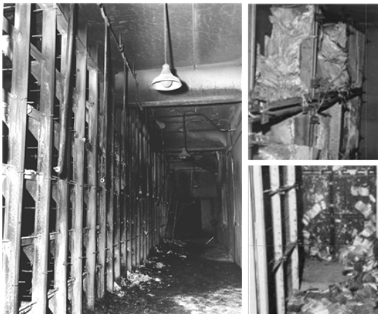
Fig. 1. Damaged HEPA Filter Units from Fire [2]
