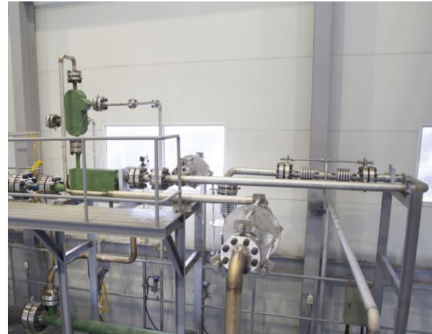
Figure 4 800HT PCHE, 316L PCHE and 4 Tied Universal Expansion Joints in HELP
