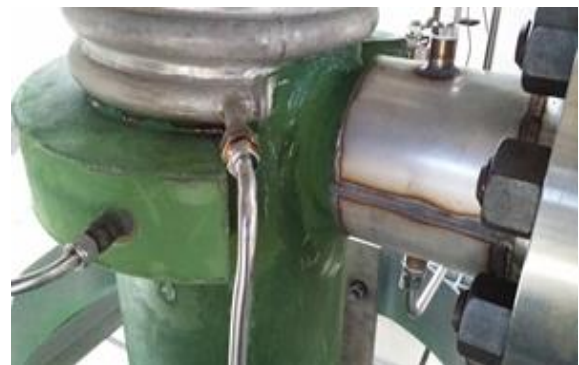
Figure 7 Water-cooled Jacket at the Outlet of a High Temperature Heater
