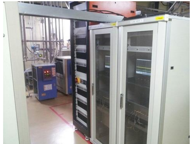
Figure 2: MEBT RF control rack
