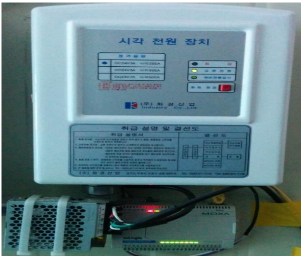
Figure 2 : Hardware of fire alarm system
