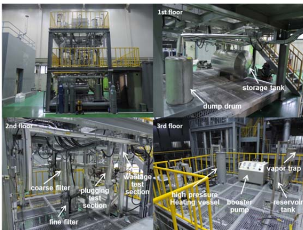
Fig. 1. Facility for the sodium-CO 2 interaction test (A booster pump and a high pressure heating vessel were added on 3rd floor recently).
