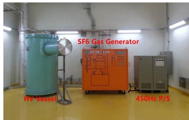
Fig. 2. High voltage power supply fabricated at KOMAC site
