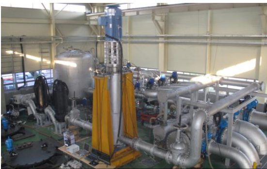
Fig. 4 Pump performance test facility with water
