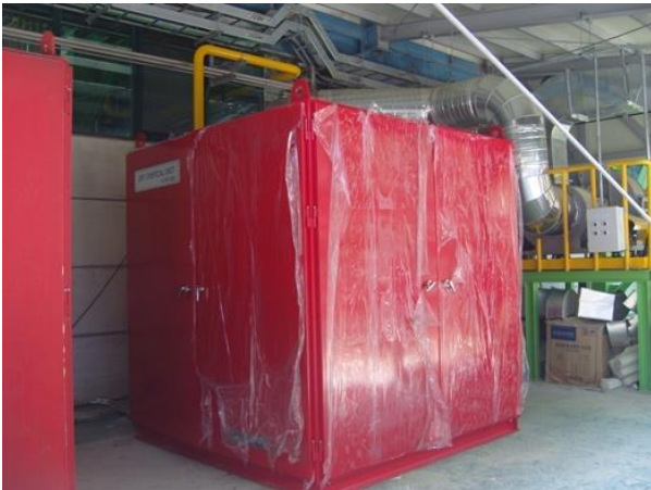
Fig. 2. Dry chemical extinguishing agent tank installed for STELLA-1
