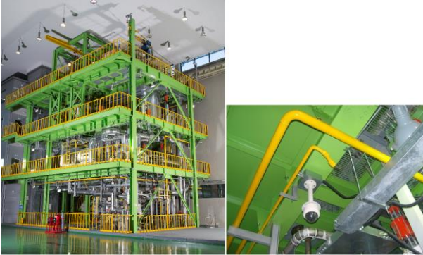
Fig. 1. STELLA-1 facility and fire extinguishing pipe line(yellow line)
