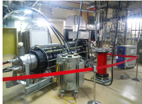
Figure 1: Installed klystron (for RFQ)
