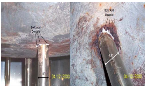
Fig. 1. Boric Acid Deposits Adjacent to BMI Nozzles #1, #46 [1].
