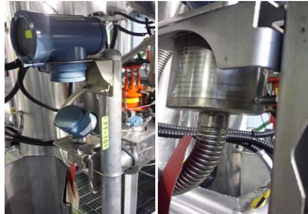
Fig. 1. The flowmeters installed in STELLA-1 facility
