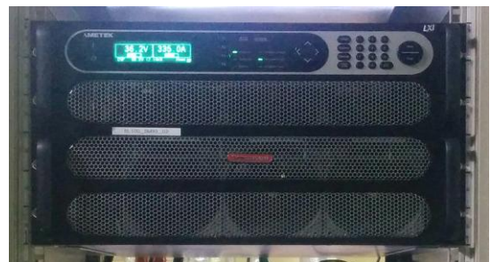
Fig. 4. The power supply for RI beam line magnet The power supply has an ethernet module and connected with KOMAC control system network. Using Transmission Control Protocol (TCP), the current
