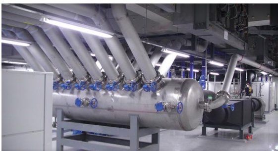
Fig 2. Cooling Header line
