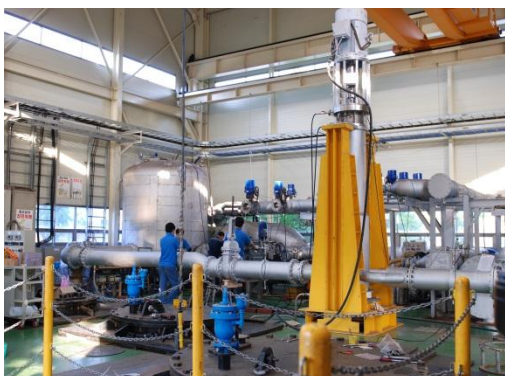
Fig. 3. Photograph of pump performance test facility with water environment
