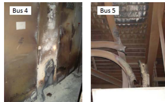
Figure 1. Damaged Electrical Cabinet and Conduits
