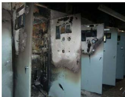
Figure 2. Damaged cabinets by HEAF incident
