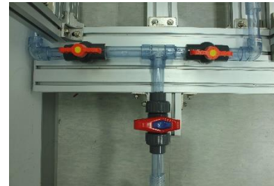
(b) Bypass valve
