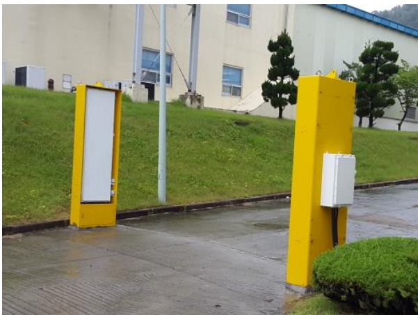
Fig. 1. A typical radiation portal monitor developed by Korea Atomic Energy Research Institute and comprises sensor panel made of PVT and NaI.
