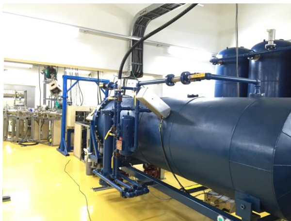
Fig. 6. Installed accelerator at KOMAC
