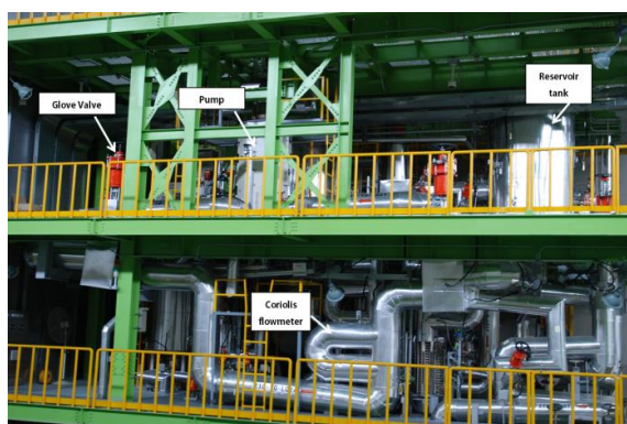
Fig. 3. Photograph of closed pump performance test loop installed in STELLA-1
