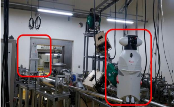
Fig. 4. The laser tracker installed for neutron beamline magnet alignment
