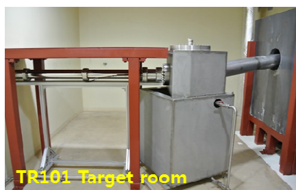
Fig. 5. Installation status in the target room
