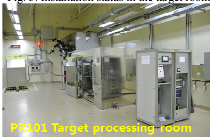
Fig. 6. Installation in the processing room
