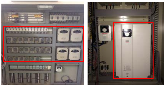
Fig. 8. Thyristor power regulator (left) for line heater control and inverter (right) for blower control in local control panel
