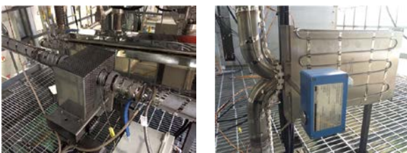
Fig. 4. Electromagnetic flowmeter (left) and Coriolis flowmeter (right) installation at sodium side
