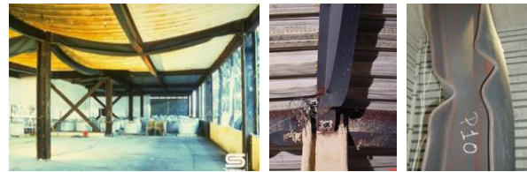
Fig. 14. Typical sagging and creep failure of structural steel
