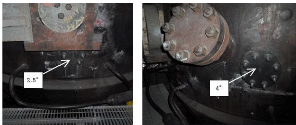
Fig. 6. Steam Generator Hand Holes
