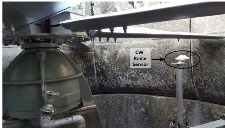
Fig. 2. Measurement setup of the RPM of the HANARO cooling tower fan. The CW radar sensor operates at 24 GHz (K-band), and it was temporarily installed for the experiment.
