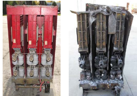
Figure 4. Rear view of breaker
