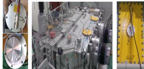
Fig. 5. UHF Sensor Attached on the Transformer [9]
