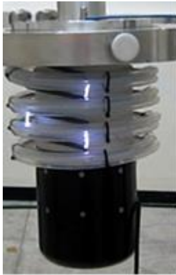
Fig. 7. Through the edges of the dividing resistors, a break-down occurred at 94 kV in the air.
